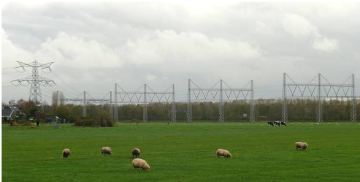
Figure 7. A 380 kV line, with lowered conductor wires hanging from portals in one horizontal plane to minimise collision risk for Great Cormorant ( Phalacrocorax carbo ), Eurasian Spoonbill ( Platalea leucorodia ) and Purple Heron ( Ardea purpurea ) daily passing this stretch of line while commuting between the breeding colony and foraging areas, Muiden, the Netherlands (Photo: Bureau Waardenburg).
