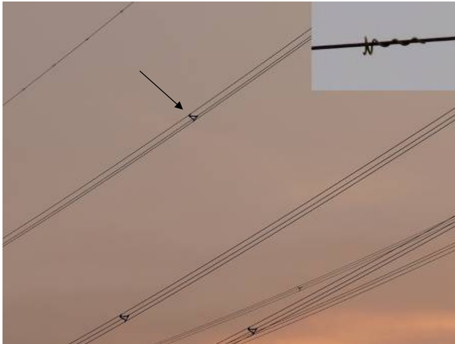
Figure 6. High voltage (380 kV) transmission line with spacers (arrow) to keep individual energised phase conductors in each bundle apart. The single thin wire in the top left corner of the photo is the ground wire (also called neutral or earth wire) that is mostly positioned above the phase conductors. In this case the ground wire has been equipped with small spirals (so called pig tails, see inset) to make this wire better visible to birds (Photo: Bureau Waardenburg).
