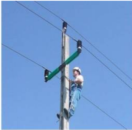
Figure 4. Cross-arm insulation carried out in Hungary (source: Horvath et al. , 2011).
